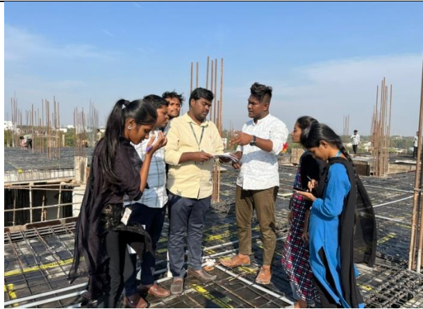
Mr. S. Hemanth Sai, Asst Professor explaining about the reinforcement details in slab
